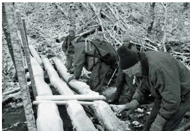
Howard McDonald, Allan Frank, Boyd Brasington and Jack Thomas build a bridge on a snowy day.
