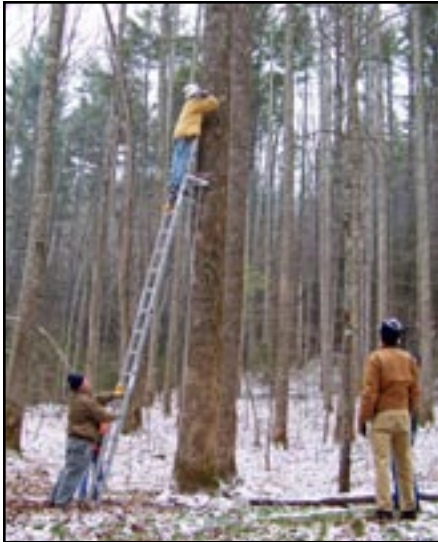
Piet Bodenhorst holds the ladder while Jeff Dektor installs cables. Photos by Howard McDonald.
